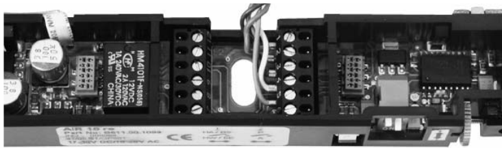
Connection terminals for AIR16
