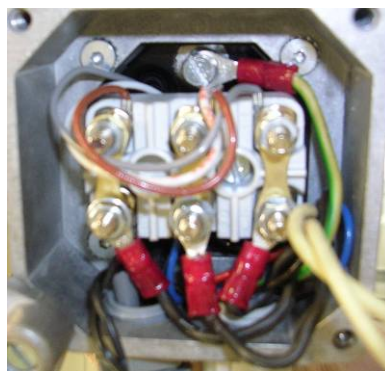
Motor (cable No.:16)
