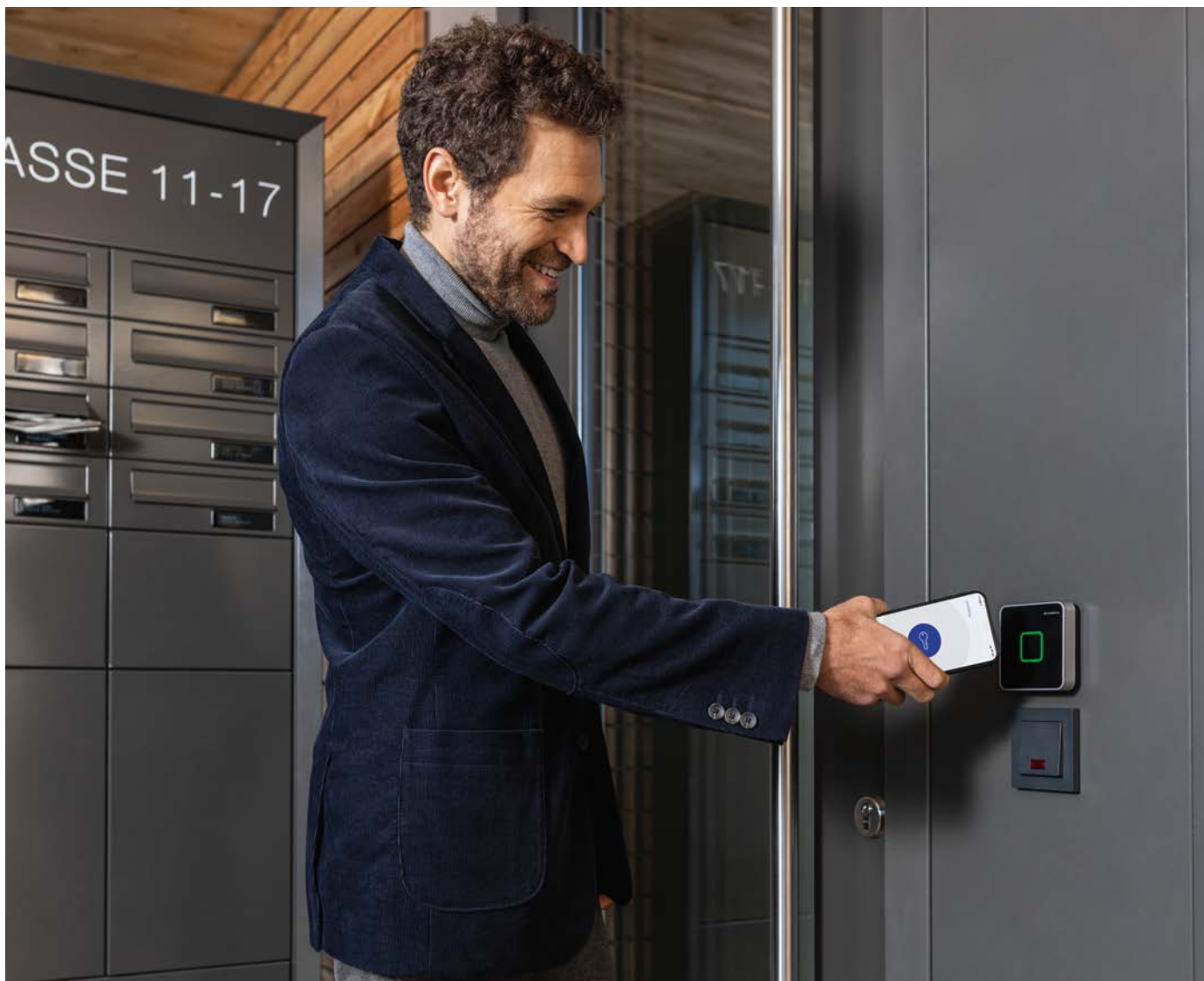
04 Online readers are installed at the four main entrances and the access to the underground car park.
