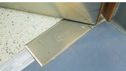
Floor spring in-situ
