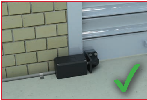
Lock mounted to the ground.
